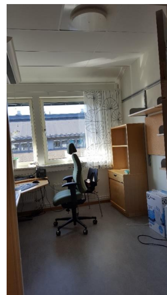
Picture 2: View of an inlet air device in an office
